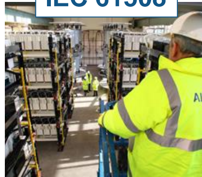
Alstom Grid UK HDVC Power Systems
